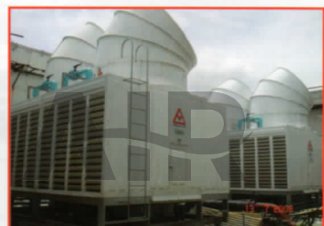
CMS-600S X 2 SETS (INTERNAL PIPING) SRIJULSUP TOWER
