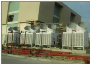
CMS-400M (C2) X 4 SETS COLGATE-PALMOLIVE (THAILAND)
